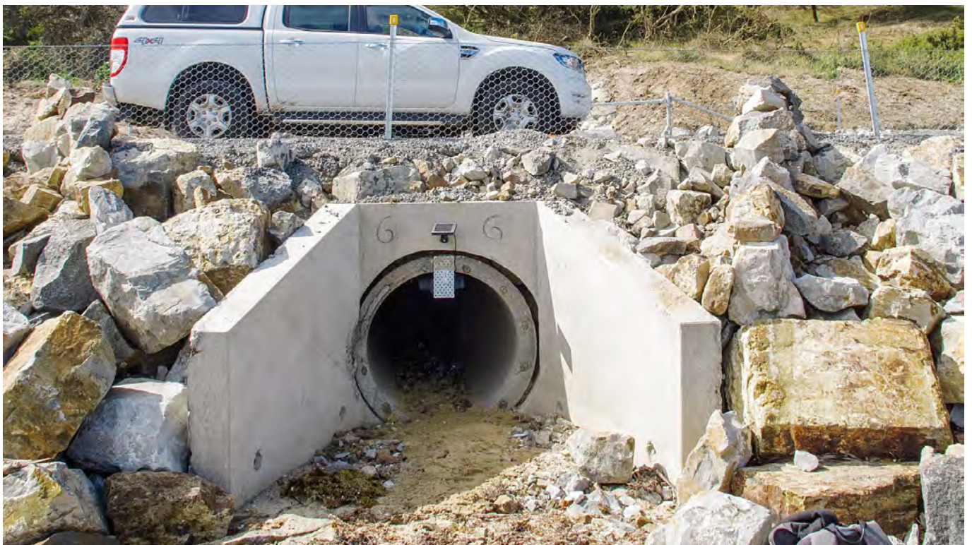
Figure 8: Photograph showing the rocky 'guides' that were constructed from the roadside fence line to the culvert entrances on the rip rap to divert penguins from the fence line to the culvert entrances on the d'Entrecasteaux Channel side of the road. Photograph ©2018 Peter Vertigan
