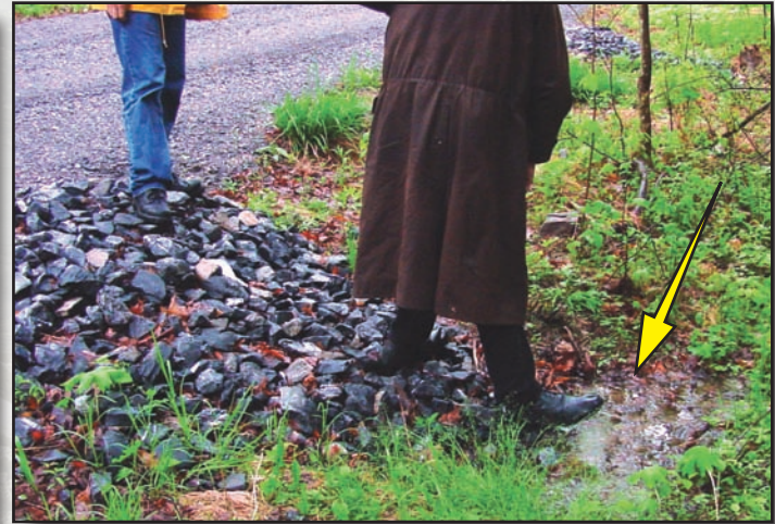
Figure 2.14—This is the same mattress outlet after completion. Notice the water flowing out of the mattress below the road.
