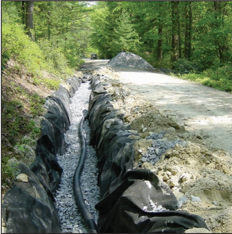
Figure 2.5—This drain collects water from springs and seeps under the road ditch.
