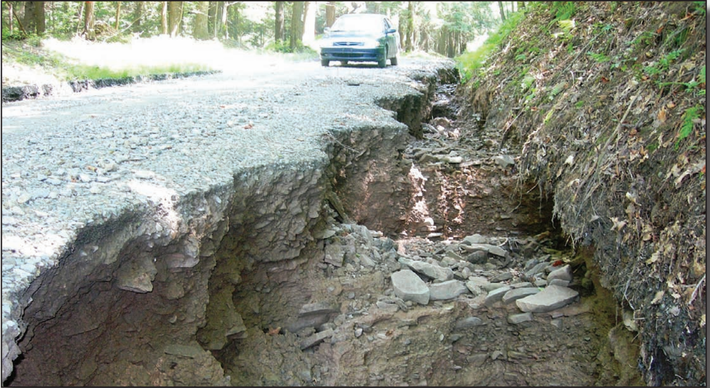
Figure 4.1—Eroded ditch caused by excessive volume and velocity of water.
