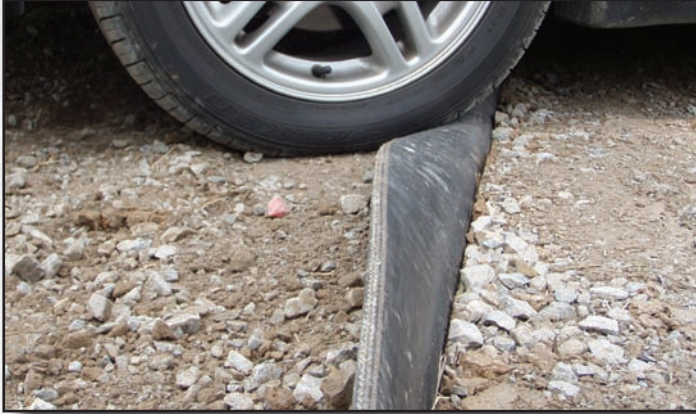
Figure 3.14—On most roads a completed diversion should leave no more than 4 inches of belt exposed.
