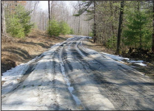
Figure 8.2—Rutting due to excess clay content.
