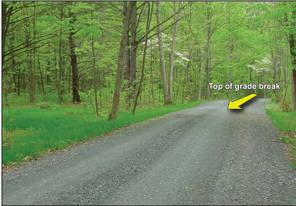
Figure 3.8—A grade break, such as the one pictured in the distance, should be big enough to shed water, but gentle enough to allow traffic passage.
