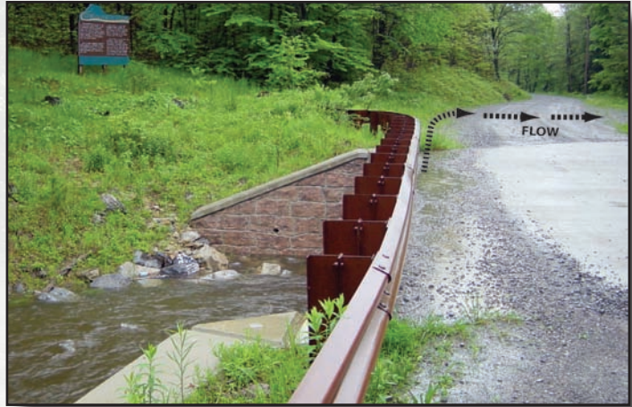
Figure 4.22b—After: Material has been added and the ditch has been reprofiled to drain away from the stream through a new cross pipe and into the woods.
