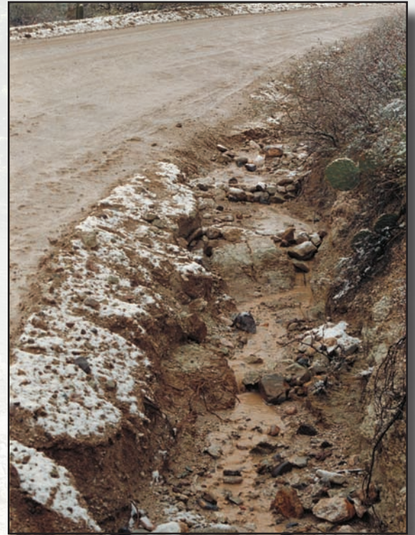
Figure 4.6—Eroded ditches are a common problem.
