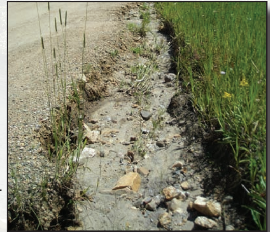
Figure 4.19—Unstable ditch. This ditch presents a safety, maintenance, and environmental concern. It is too deep, too wide, unvegetated, and can route sediment to the stream.
