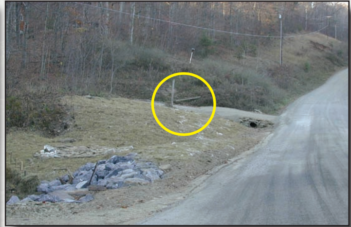
Figure 7.14—The broad-based-dip on this driveway provides a good transition and keeps water off the public road.
