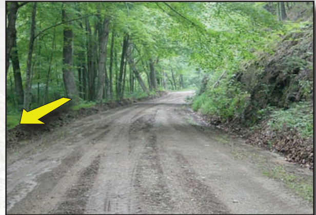
Figure 4.15—The berm was created by recent grading. Removing the berm and crowning the road allows sheet flow into the vegetation to the left.
