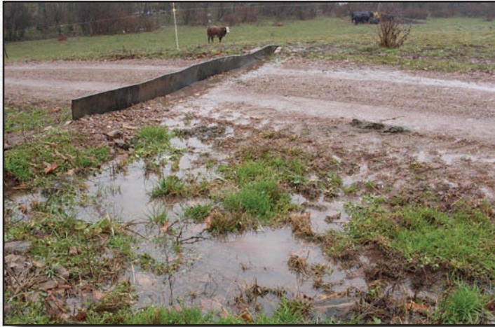
Figure 7.13—This conveyor-belt diversion on a farm access lane prevents drainage from flowing on to the public road at the bottom of the hill.
