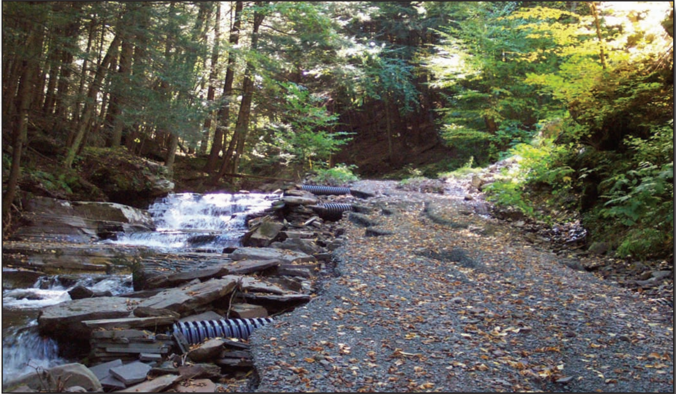
Figure 6.1—Consequence of poor road location results in loss of road and increases sediment delivery.
