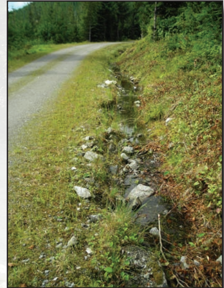
Figure 2.4—Road ditch with standing water.
