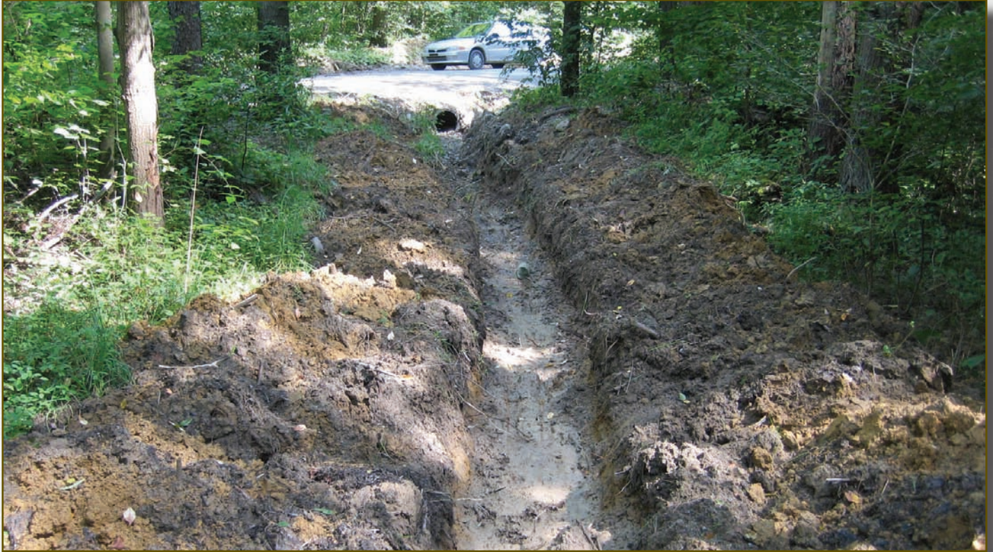
Figure 5.1—Culvert placed below the natural elevation requires frequent maintenance and long ditch outlets.
