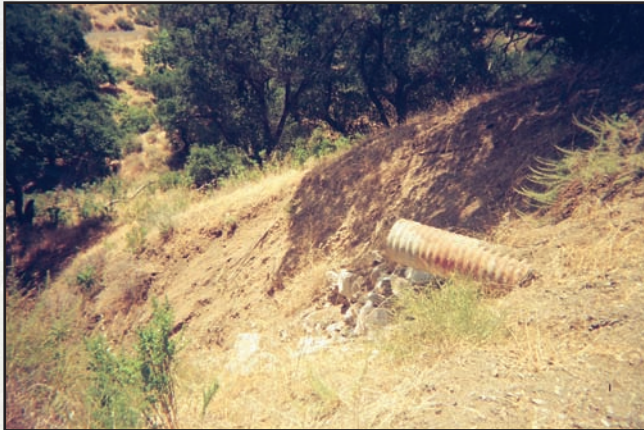
Figure 5.2—Shotgun culverts causes accelerated erosion.
