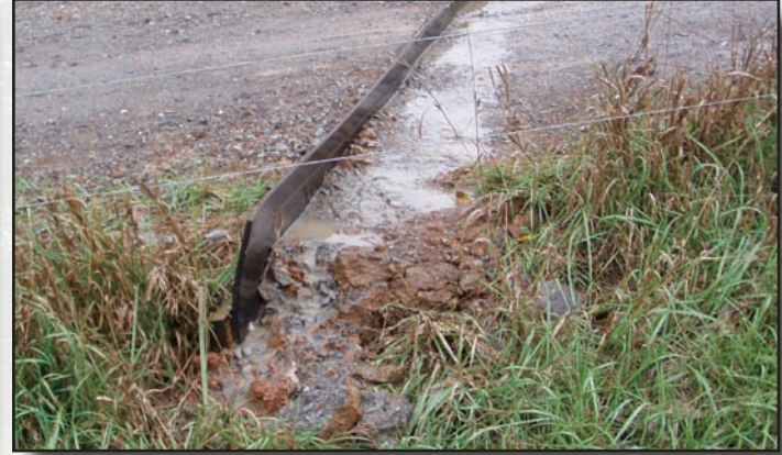
Figure 3.15—A completed diversion directs surface drainage off the roadway and into a field.
