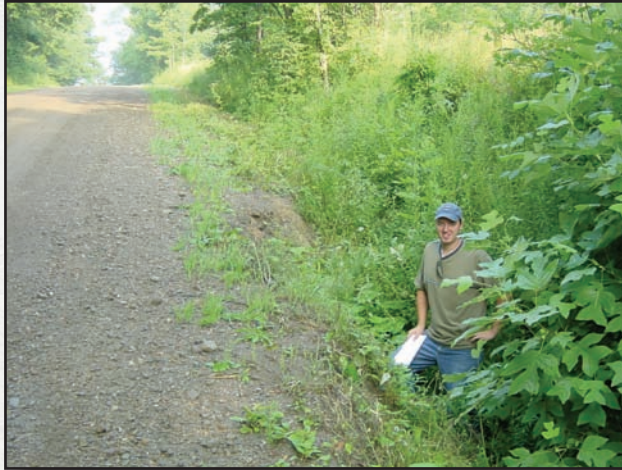
Figure 4.2—This photograph is taken only 300 feet from the top of the hill, yet the road ditch is over 5 feet deep. Further investigation of the site revealed a large amount of water emptying out of a meadow and into the road ditch. This water should be either diverted before it reaches the road or handled as quickly as possible and not allowed to flow down the road ditch.
