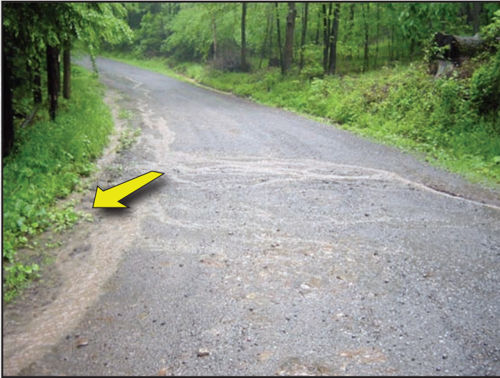
Figure 4.14—Berms can range from several feet high to only a few inches high as pictured here. The small partially vegetated berm on the left is preventing runoff from exiting the road surface. A stable vegetated buffer exists to the left, but the berm is causing an unnecessary ditch to form at the road edge.
