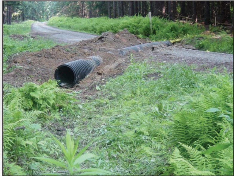
Figure 5.7—A shallow cross pipe being installed: The cross pipe shown is partially installed. Notice that the pipe outlet is at the elevation of the existing ground, no outlet trench or tail ditch is required. The top of the pipe is ABOVE the existing road surface. The required pipe cover is obtained by importing fill. When completed, the fill will create a grade break over the pipe.
