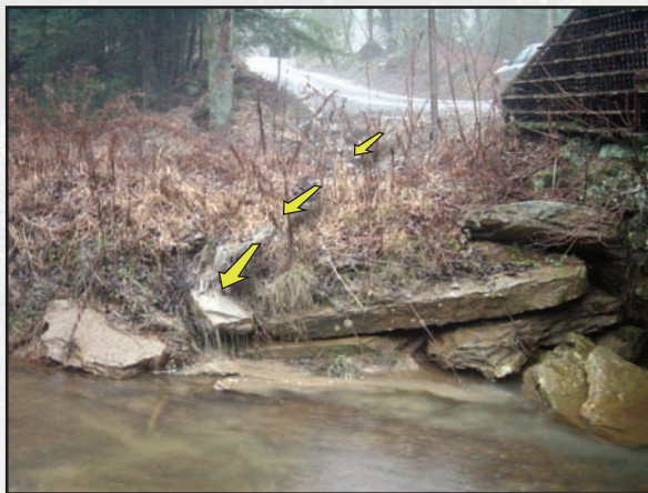
Figure 4.20—Traditional urban stormwater approaches collect and convey ditches directly to streams, as pictured above. Modern rural stormwater management should disconnect the road and stream by avoiding concentrated discharges to streams and encourage drainage dispersal.
