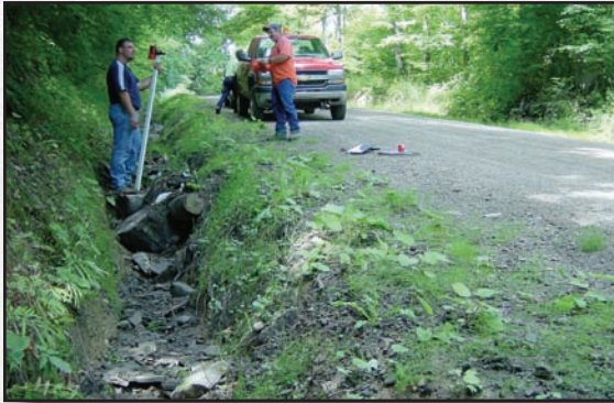
Figure 4.4—This eroded ditch is a symptom. The problem is excessive water volume for this road gradient and soil, and must be managed upslope.
