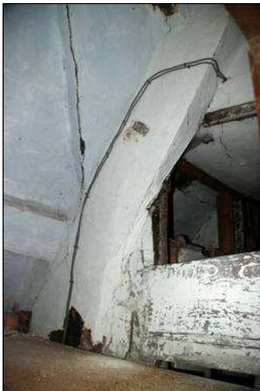
Plate 51: Join between Truss 4 and the partition over the stair well, looking north
