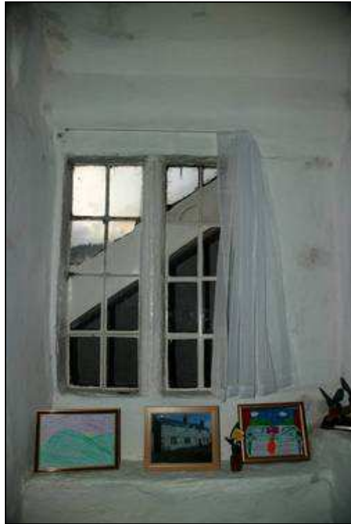
Plate 17: Obstructed window at the head of the stairs, looking NW
