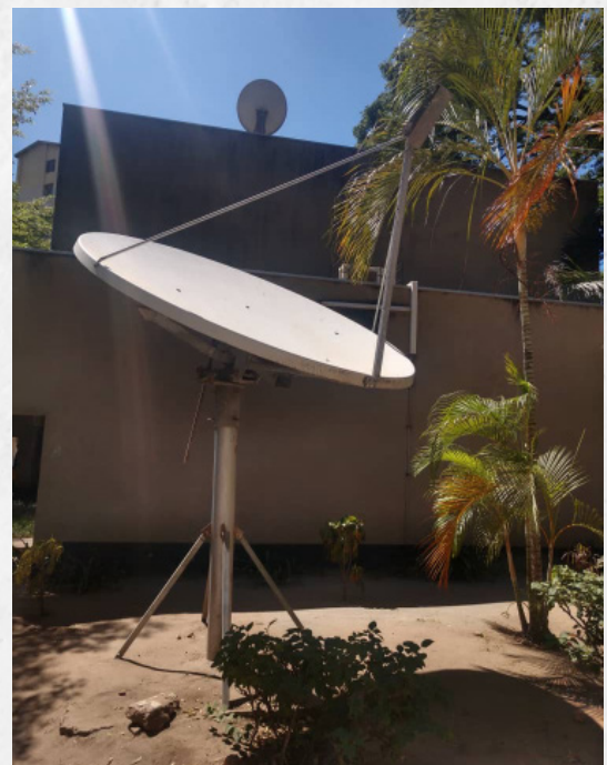
Telecommunication Transmission dish at DIT installed by the Company
