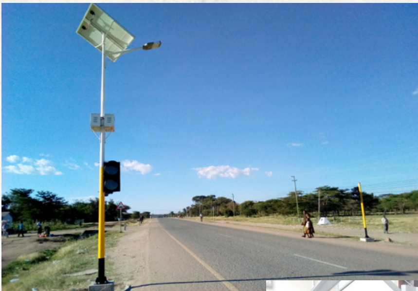
Street Lights installed by the Company at Bariadi Simuyu
