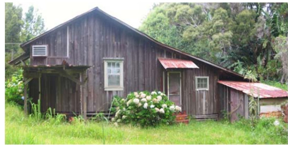
Photo 3-6. Historic Rating: 5 Very Poor Condition Pu‘u ka Pele, TMK: 1-4-02: 76
