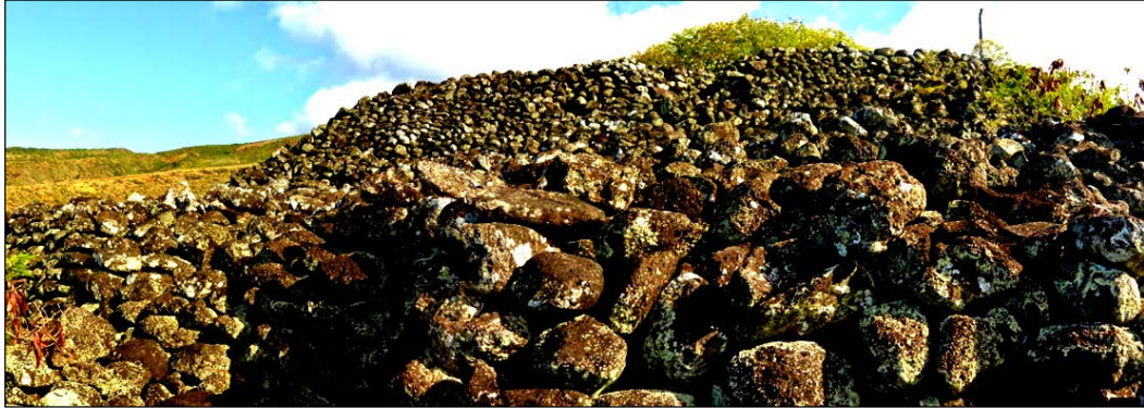
Figure 37. Recent photograph of Kahokukano Heiau showing condition of retaining walls at this site (photo from Google Earth).
