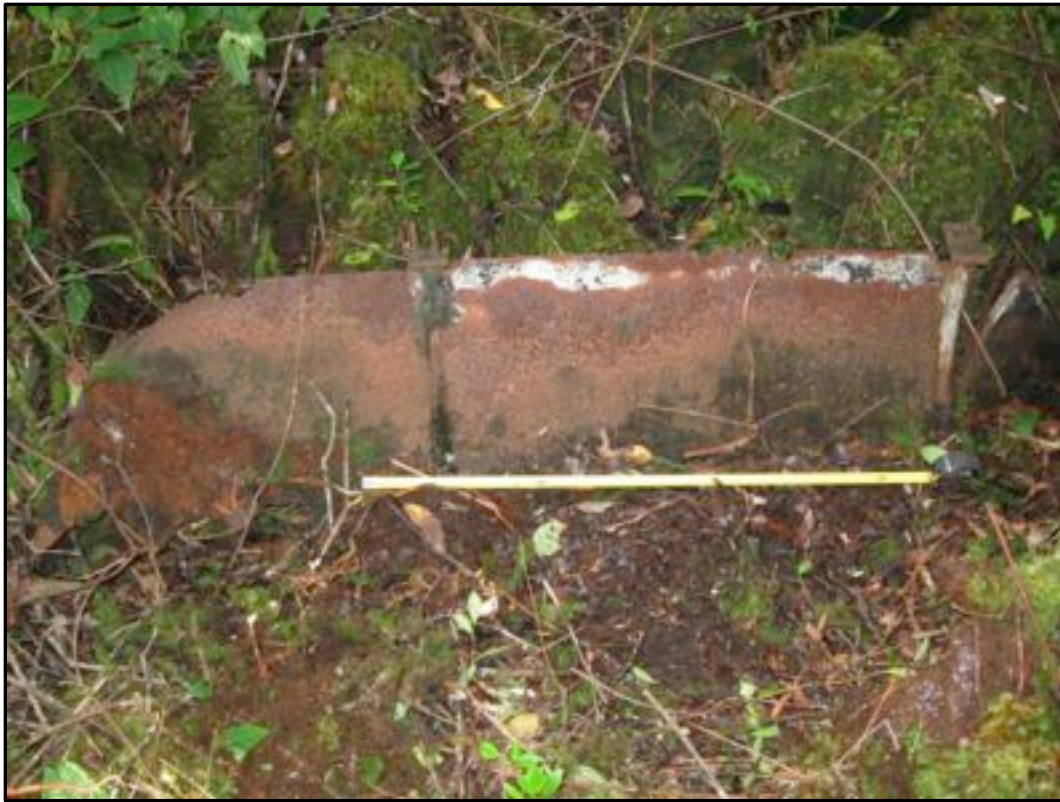
Figure 70. Displaced remnant of Site 20870 Flume in Block 12 (view to northeast)
