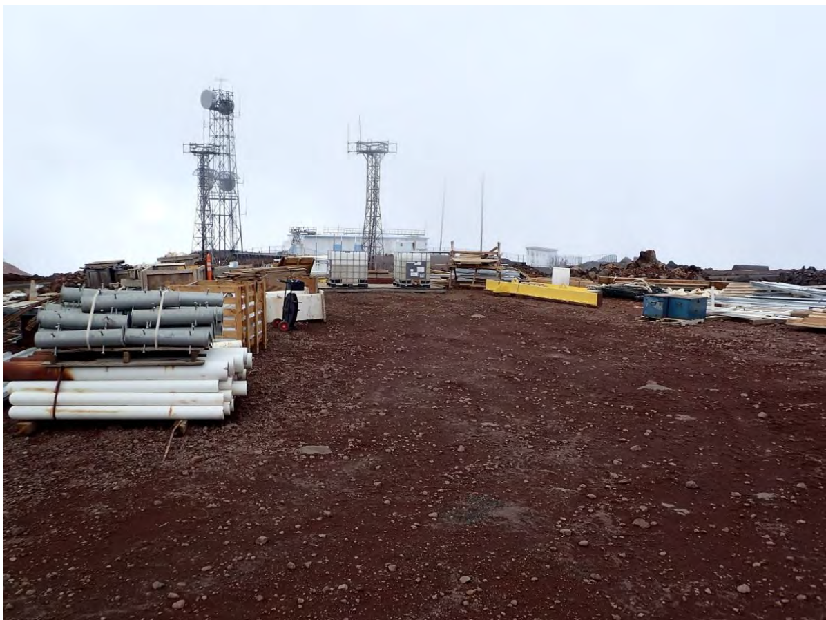
DKIST storage and staging site near the FAA facility was clear of wind-blown debris.
