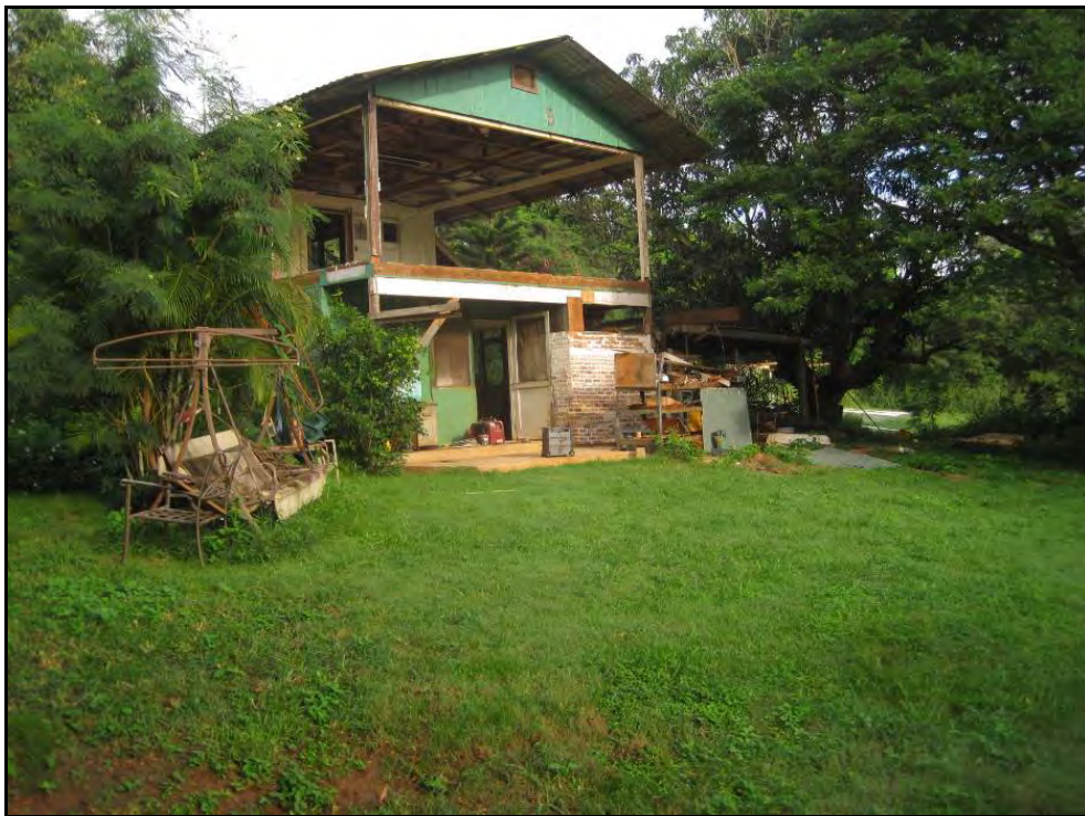
Figure 120. Buildings on the Cash Ranch property ready for demolition, view to northwest
