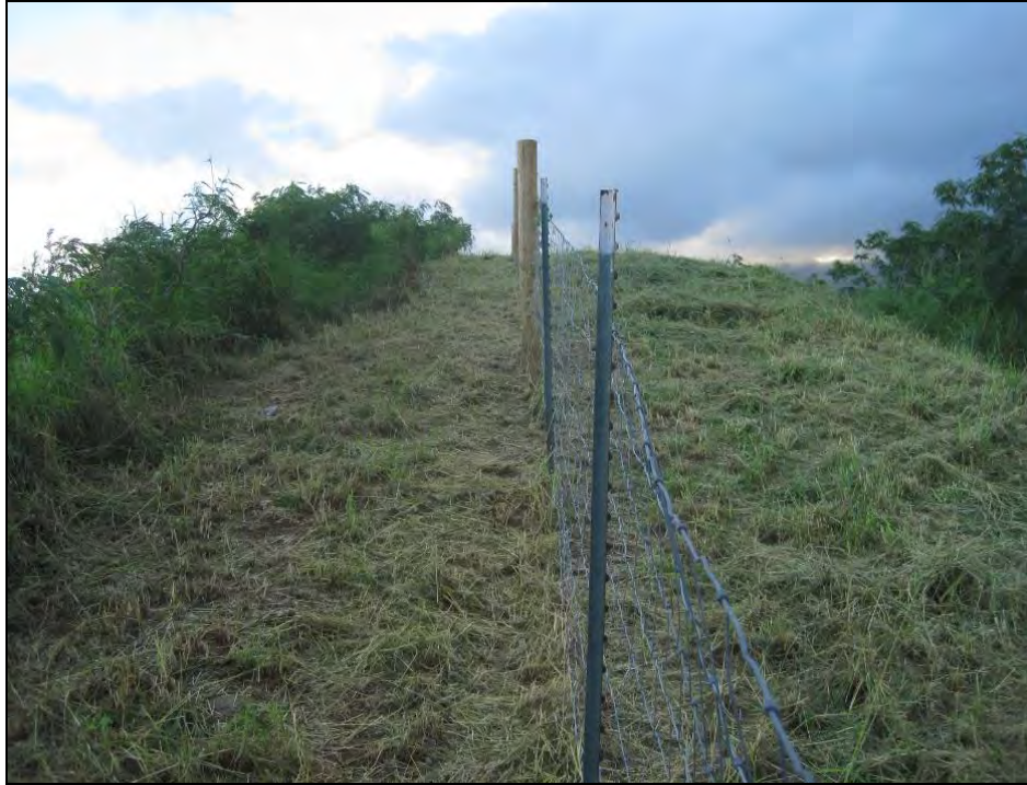
Figure 73. Recently installed wire fence marks the property line between the State and private property in the eastern portion of the ridge, view to west
