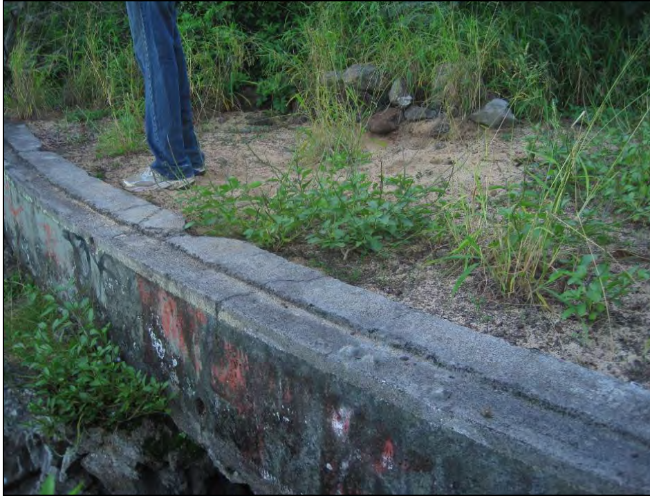
Figure 71. Concrete platform for a former reservoir with sand in the center of structure, view to southeast
