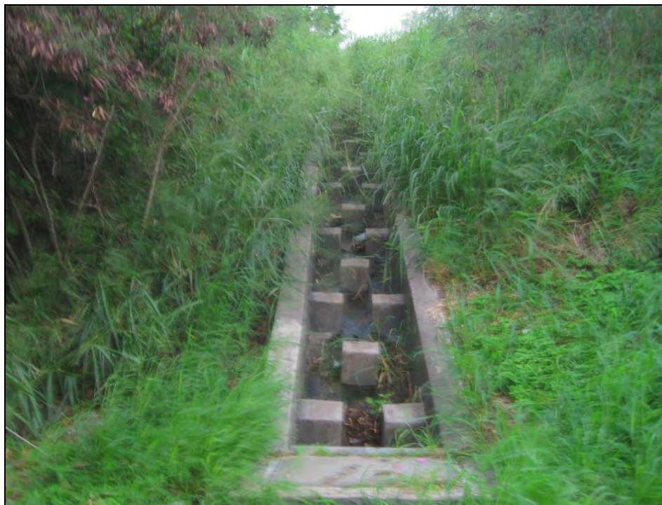
Figure 70. Drainage ditch extending uphill from Kailua Road to the beginning of the Pu‘u o ‘Ehu ridge trail, view to east
