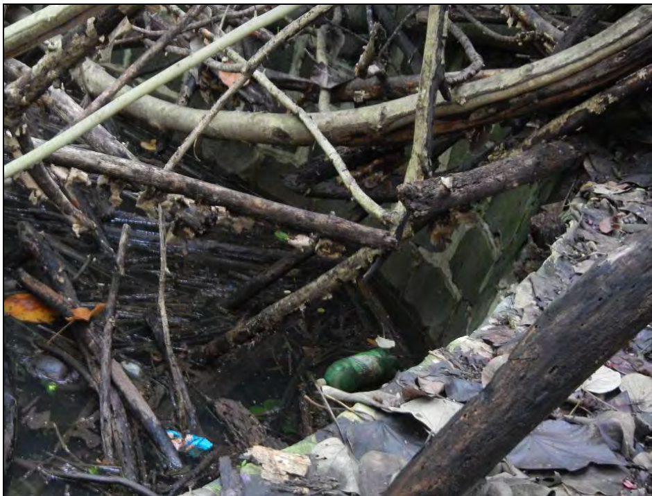
Figure 88. SIHP # 50-80-15-4042, U-shaped southern portion of the Waimanalo Irrigation System pump house, view to east
