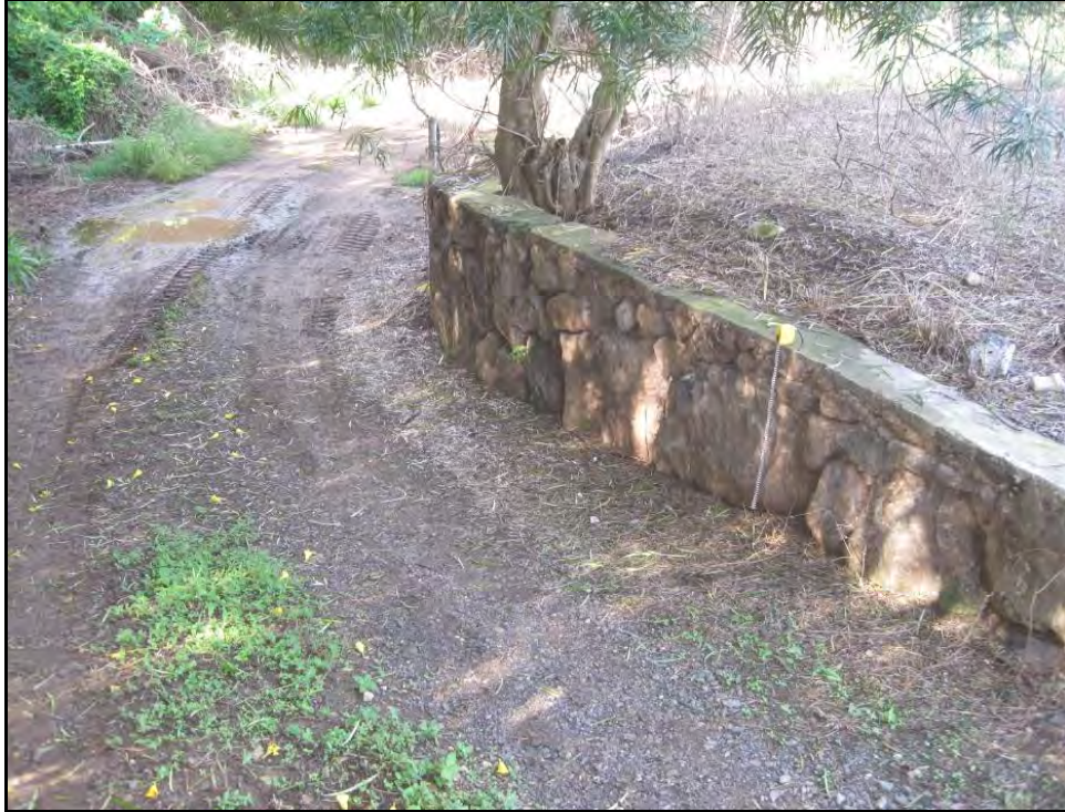
Figure 67. Basalt rock and mortar retaining wall at the DOFAW entry to Hāmākua Marsh, view to southwest
