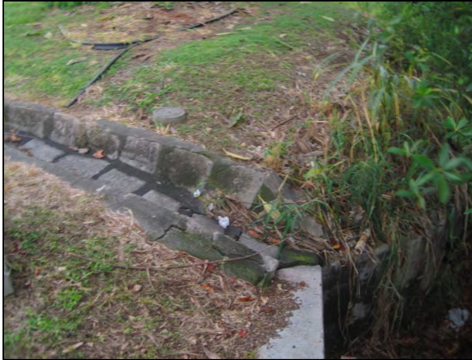
Figure 69. Drainage extends from intersection of Kailua Road and Hāmākua Drive into the north portion of Hāmākua Marsh, view to southeast
