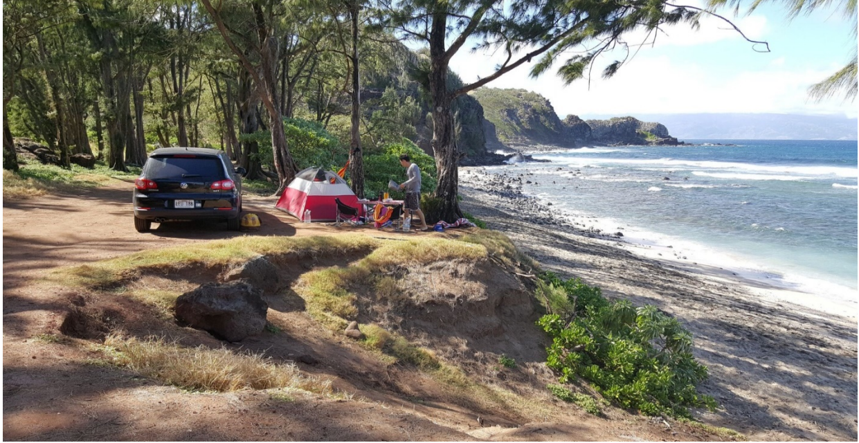
Evidence of embankment erosion at Keonehelele'i Beach.
