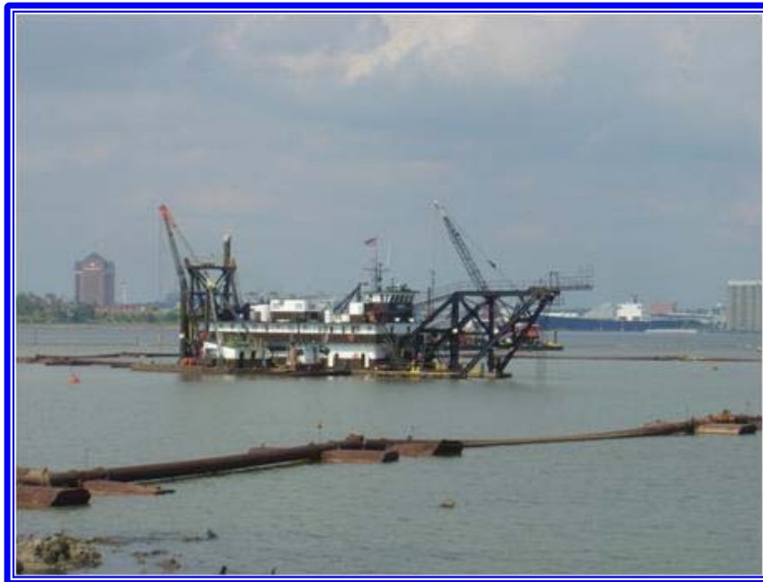
Figure 5-3. Pipeline to Transport Dredged Material
