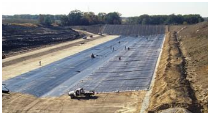
Installation of a compacted clay and geotextile liner at a landfill site in Wisconsin. Photo: DNR
