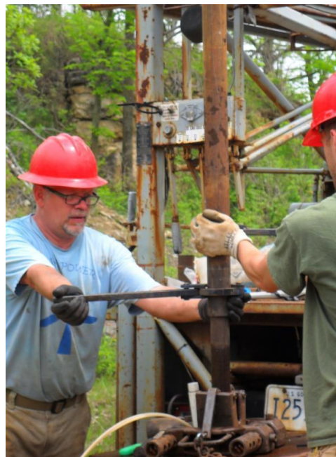
Pete Chase and Jacob Krause, WGNHS, install well casing during a WGRMP-funded experiment designed to improve understanding of virus transport from wastewater to drinking water wells. Photo: Blake Russo-Nixon.
