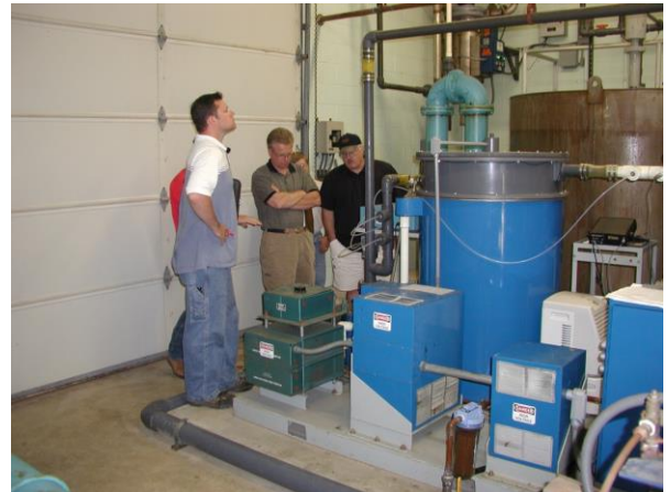
Ozone generator inspection at a public water supply system.
