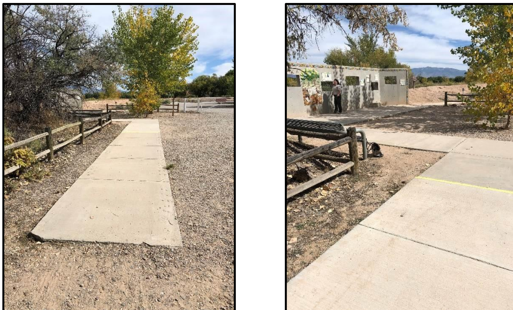
Figure 24. Existing viewing blind access at RGNCSPP parking lot to view the Candelaria Wetlands.
