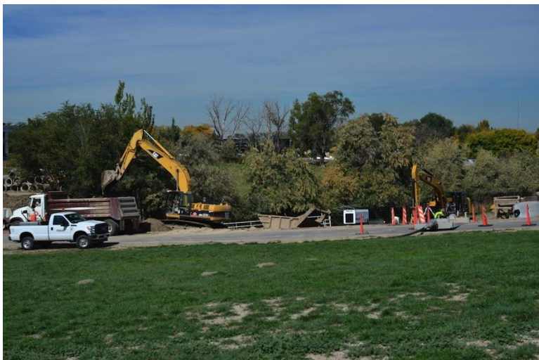
Figure 35. All too common construction impacting spring creek tributaries of the Jordan River, UT. This location at the Jordan Valley Water Conservation District property was photographed October 2014.
