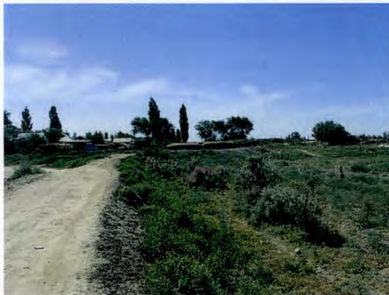
Fig. 1-2: Insufficient (?) flood protection dike at Abay village. According to reports recently constructed under SYNAS-I
