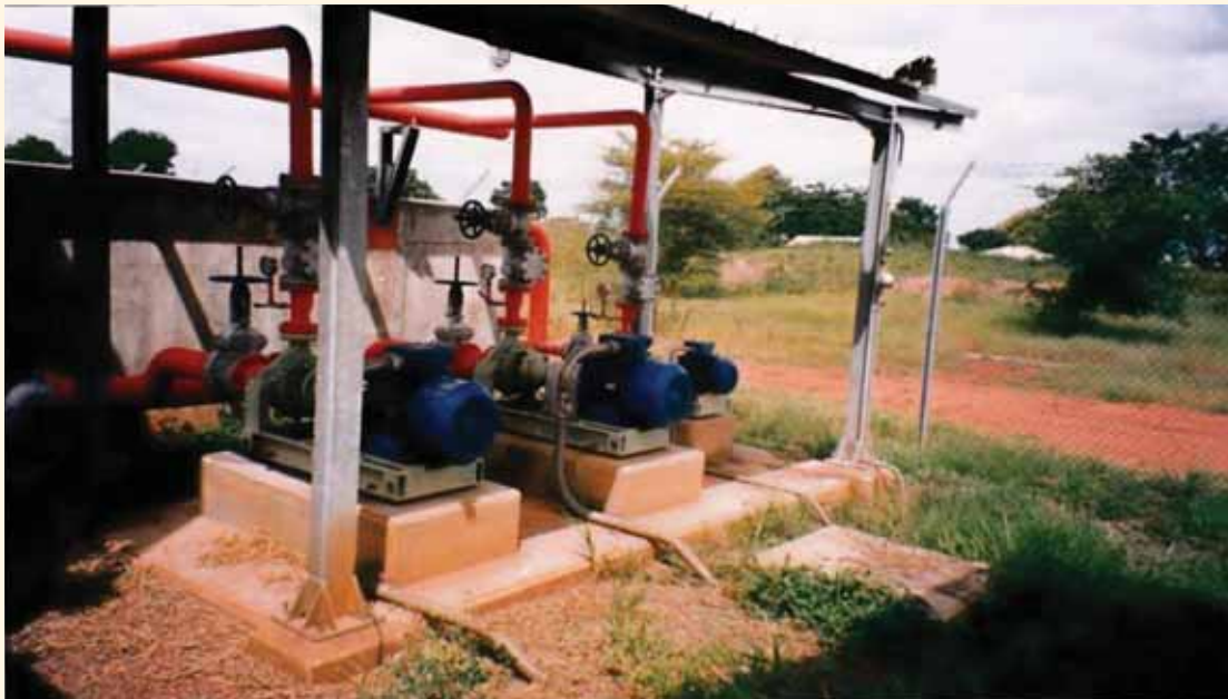
Top: 30 kV/415-240 V 315 kVA transformer station supplied from a three-phase Iliceto shield wire scheme; Bottom: associated oil pumping station. Photographed by Prof. Francesco Iliceto.
