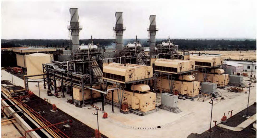
Hainan Meinan Power Company, a diesel power plant designed to respond to fluctuations in demand, will help eliminate power outages in Hainan Province, China.
