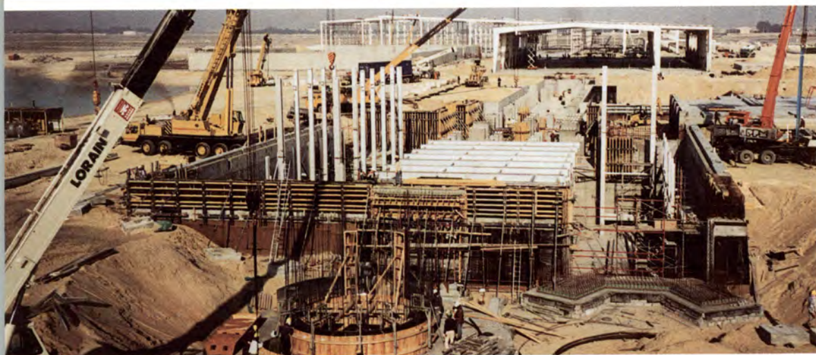
Construction is under way at Saudi Guardian International Float Glass Co., a joint venture of Guardian Glass Investments of Luxembourg and two Saudi companies.
