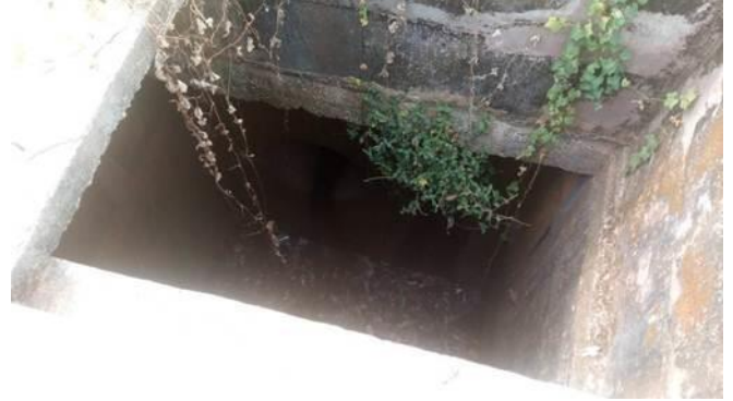
Manhole constructed by previous Interventions in Ogiso Community
