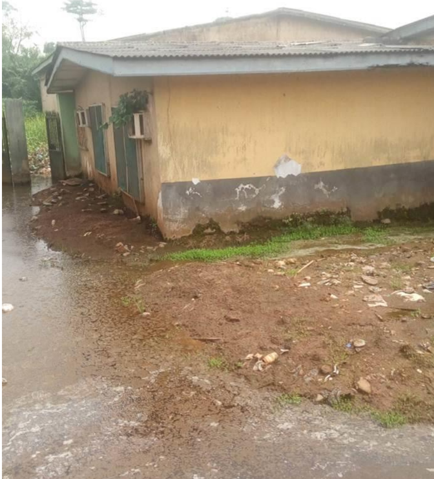
Plate 4.1: Severe erosion case in Ogiso Community
