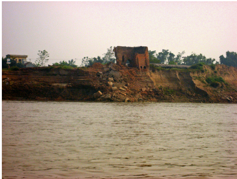
Photo 4-5. Active bank erosion Red River (7389)
