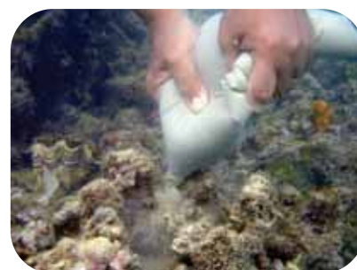
Squeezing cement and sand concrete mix (with plaster of Paris added to speed setting) from a plastic bag onto a degraded reef prior to attaching a transplant (R. Dizon). Robust plastic pastry bags can also be used to pipe cement onto substrate.
