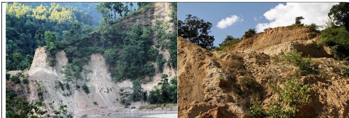
Figure 4-8: Landslide and instable slopes along NNM section.
