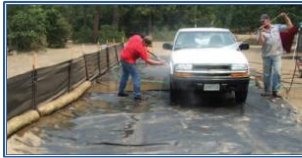
Figure 7. Contain waste water when washing vehicles to prevent spreading AIS and/or their parts
