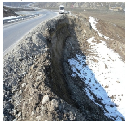
Figure 19- Flow-slide at Ch. 105+000
