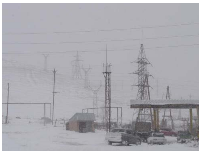
Figure 12-8: Noratuz line towards Hrazdan TPP substation
