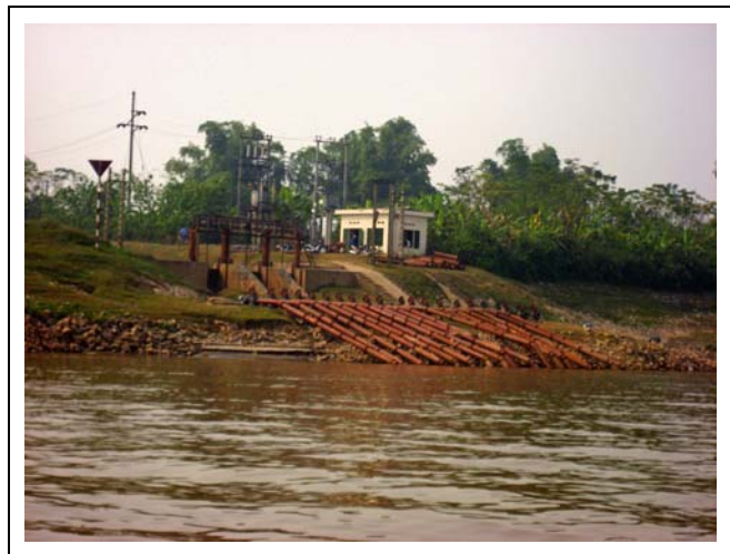
Photo 4-22. One of the pumping stations upstream of the Red River
