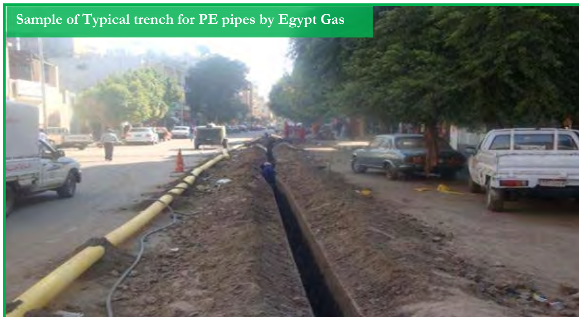
Figure 2-24: Pictures showing sample of typical trench for PE pipes by Egypt Gas
