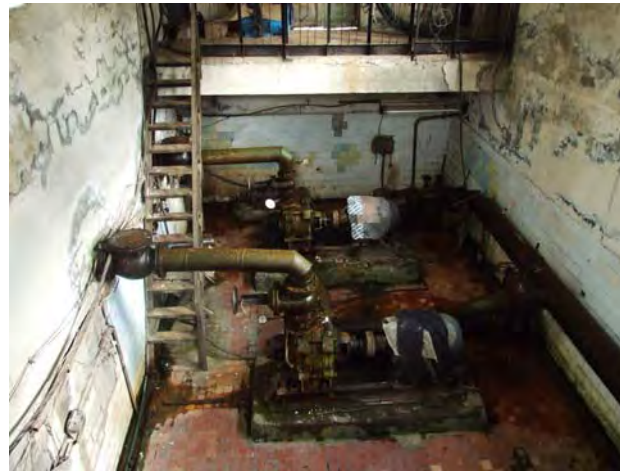
Pump station in the Reservoir site
