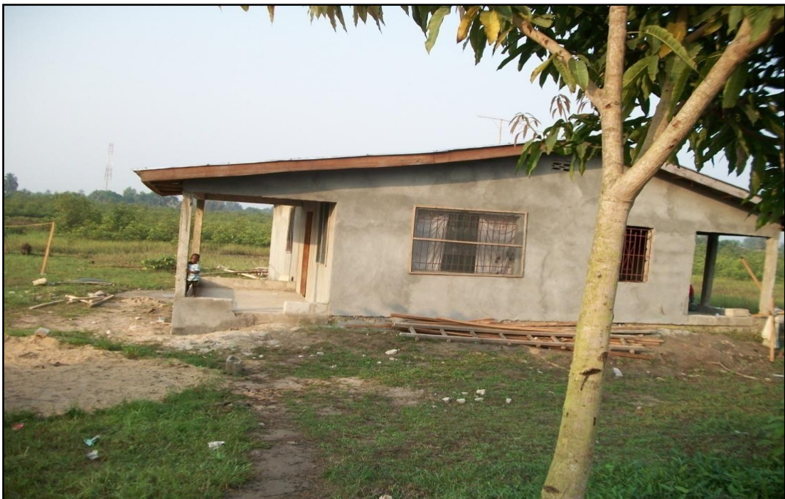
Figure 15 Sun dried bricks house near completion constructed with cement & corrugated sheet roof
