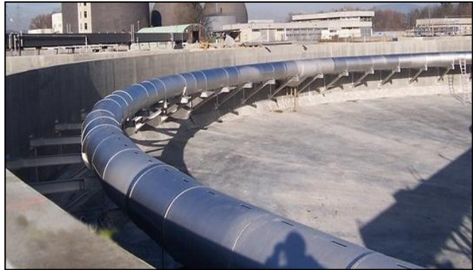
Figure 2: Effluent Pipe, Huber Technology SE
