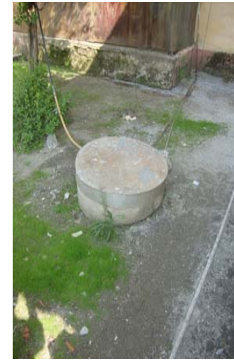
A sub-artesian well and pump manhole in a private plot
