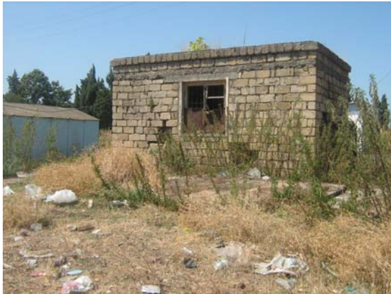
Existing drinkable Water Reservoir
