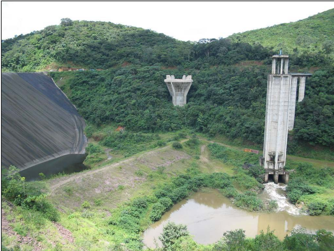
Figure 7.3.2-2: View of Upstream Face of the Dam, ‘Morning Glory Spillway’, intake and intake tower
