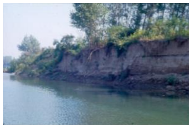
Figure 2-10: Collapsed banks on Lower Drina River
