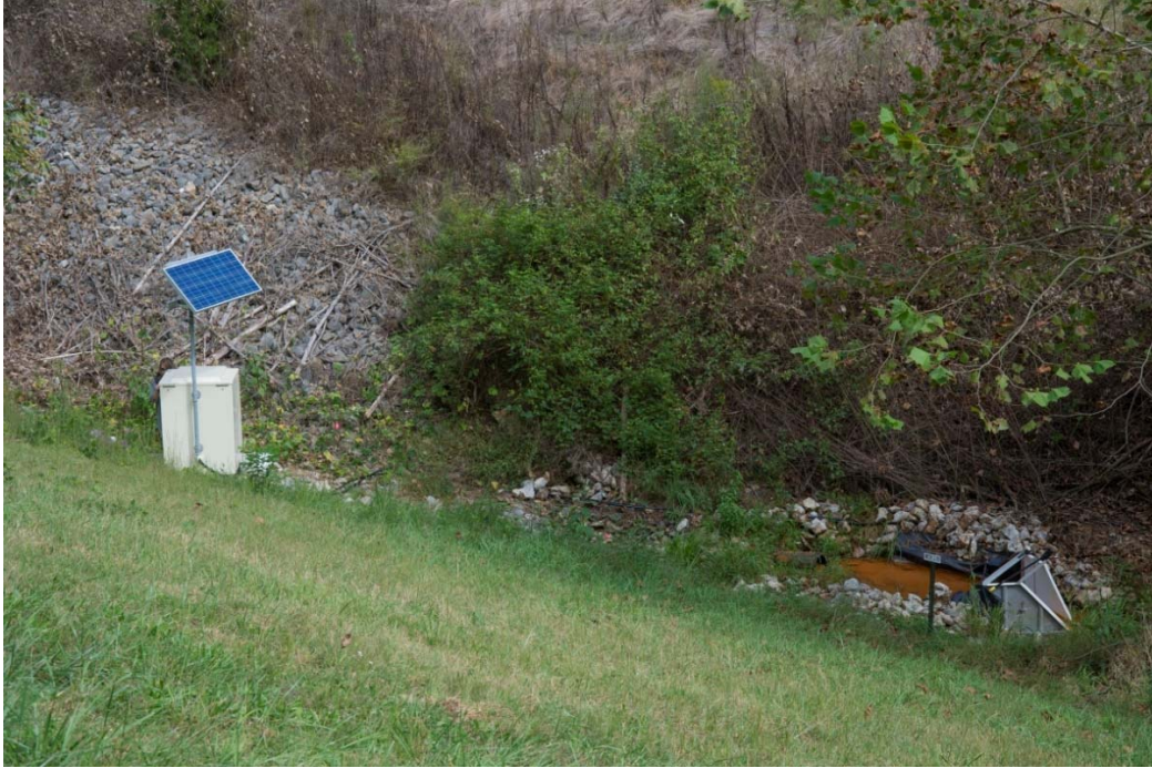
Figure C.1.3. Leachate influent (MCK 2.05) monitoring station.
