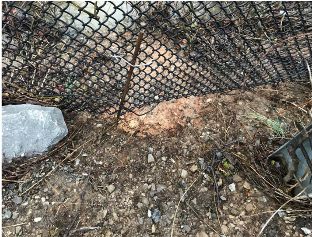
Figure 8.8. Erosion beneath the K-1007-P1 Holding Pond fish barrier fence along Poplar Creek.
