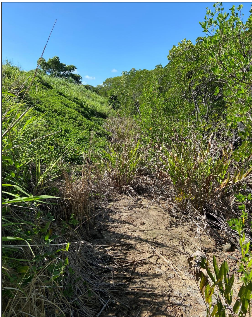
Plate 2: Steep engineered slope approx. 4-5m in height between native mangrove vegetation and the site
