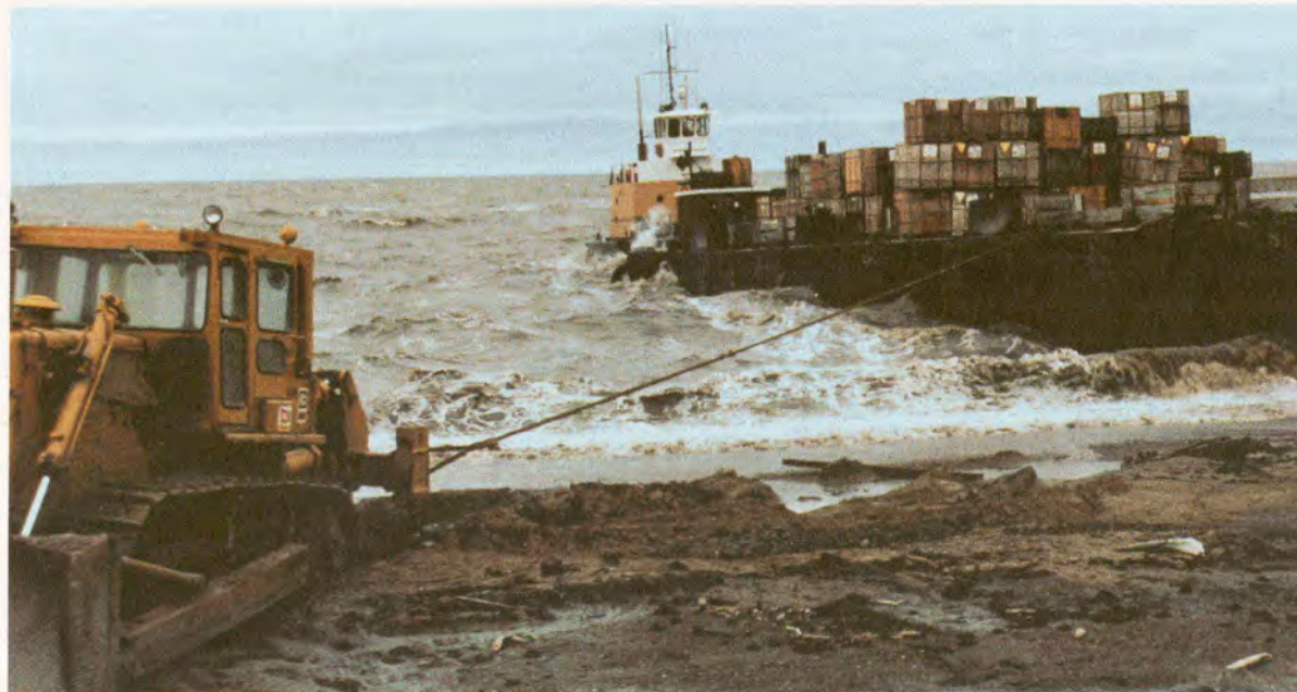
Landing barges on the coast near Camp Lonely. Shipping by barge is the most inexpensive method of transporting large amounts of material to the Arctic coast but is generally restricted to a short period in August when the ice retreats from the shorelines. Photograph by S. Krogstad.
