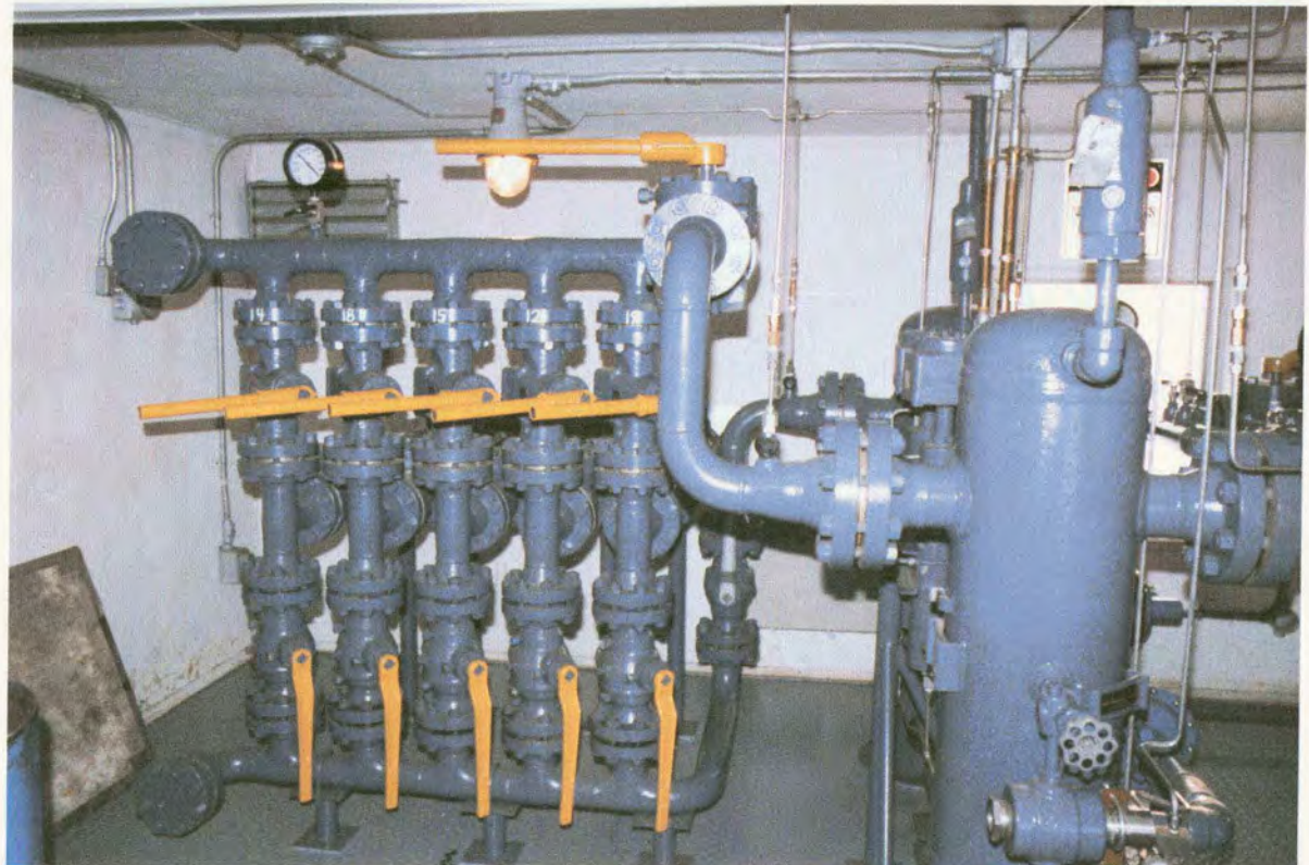
Manifold where the flowlines enter the East Barrow metering and regulation (M&R) building. Photograph by Robert Lantz.
