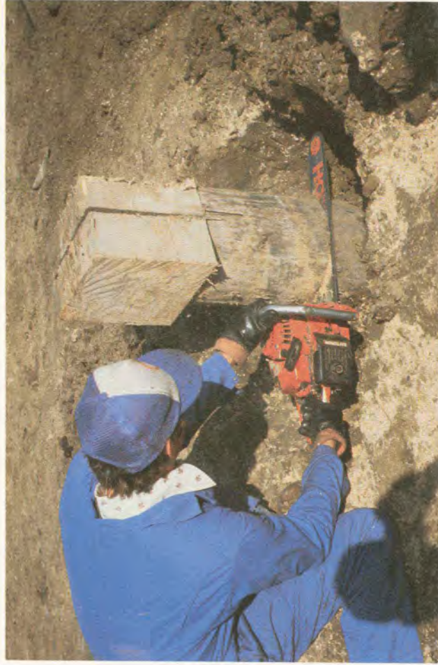
Part of the cleanup operation at old drillsites consisted of cutting off pilings, “below grade” of the drill pad. Photograph by John Schindler.
