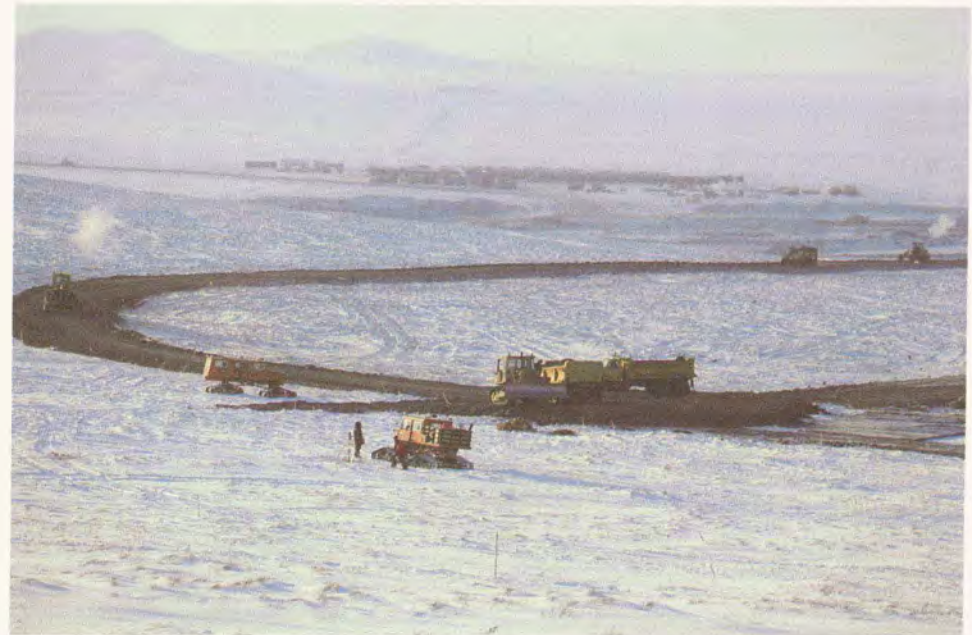
A gravel access road leads from the well site to the borrow site and all-season Herc airstrip. Photograph by Jeep Johnson.
