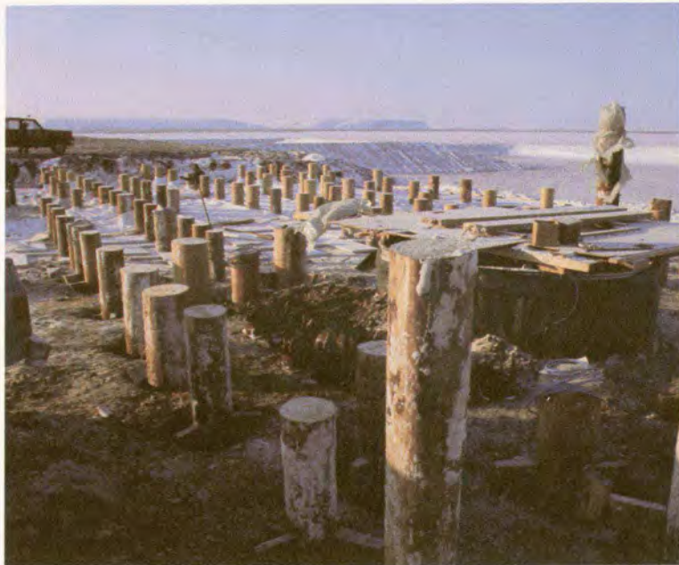
Construction of one-season thick pad at the Seabee wellsite. Photograph by Jeep Johnson.
