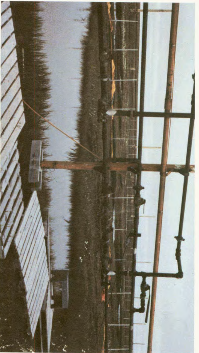
Flowlines into the central production facility in the older South Barrow gas field. Note the confusing, interconnected piping, threaded connections, and valving exposed to the weather. The South Barrow production facility and gathering system were largely built on site from surplus materials. As the number of gas wells increased, valves and pipes were added to accommodate them. The operators said "it just grew like Topsy." Photograph by David Fears.
