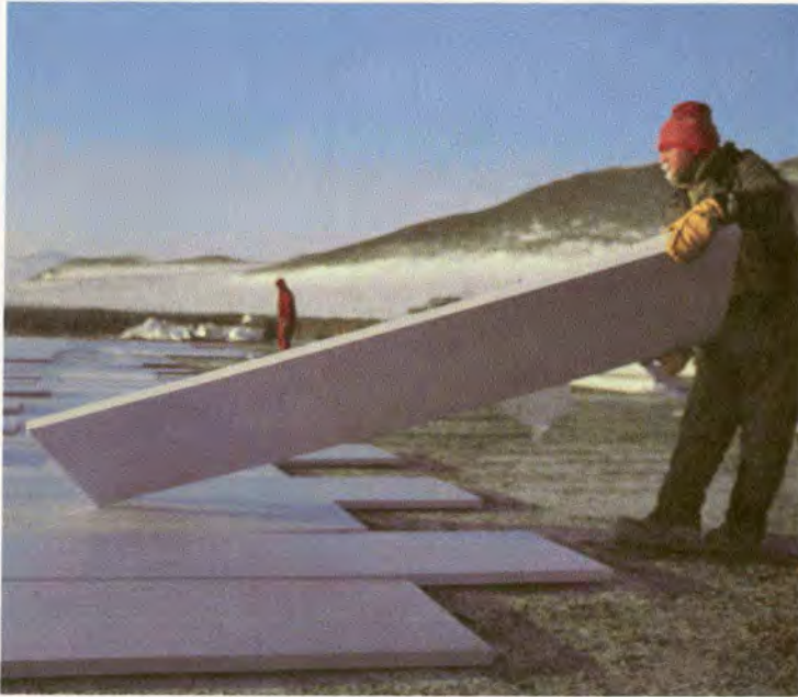
Six-inch-thick insulation protects the permafrost layer beneath the Lisburne drill pad. Photograph by Jeep Johnson.
