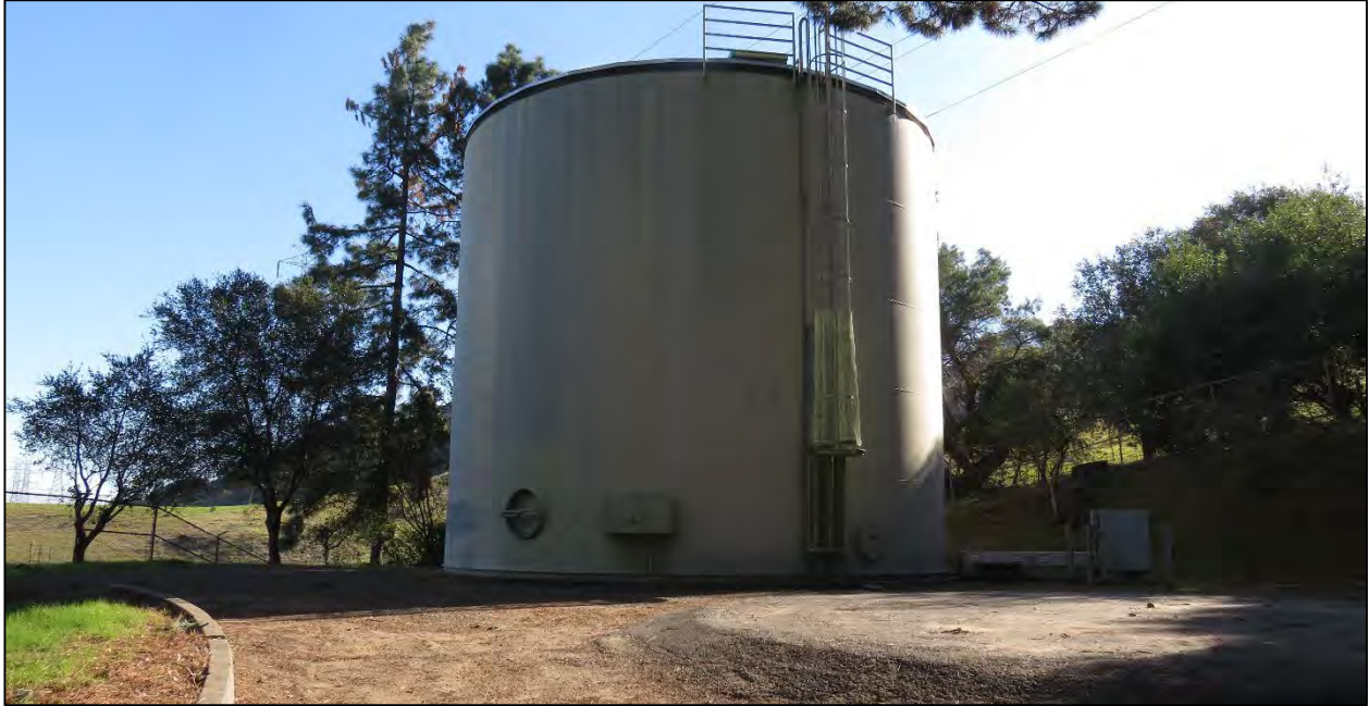
Existing Dos Osos steel-welded reservoir. View from Los Norrabos Road gate, facing south. Photo taken on December 18, 2017.
