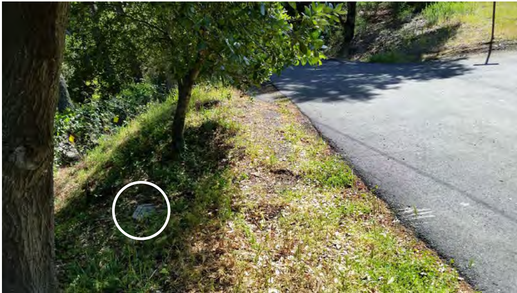
Existing 0.75-Inch Air Valve at the Intersection of Alta Vista and Lomas Cantadas within the Dos Osos Pressure Zone in Orinda
