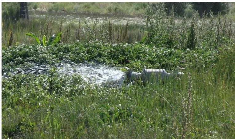
Photo 2-3. Close-up of open water valve.
