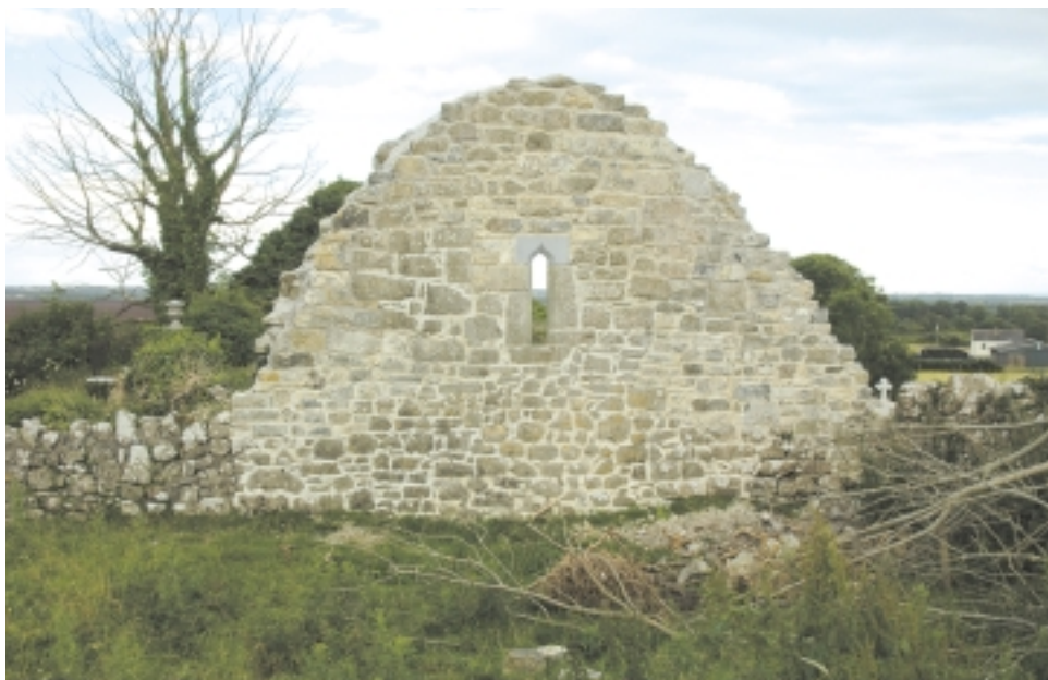
The window in the recently-repointed west wall of the former Carmelite church at English would suggest a date around the fifteenth century for much of the surviving masonry.
