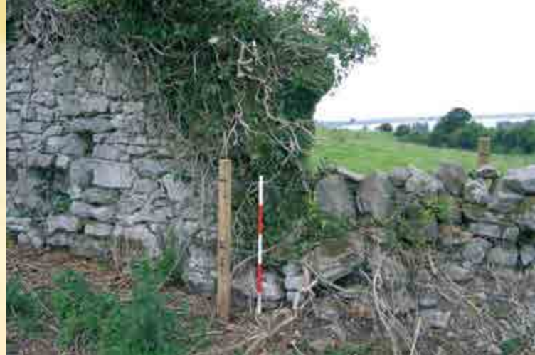
An excellently preserved stretch of original wall meets a rebuilt stretch. Note the 'letterbox aperture' on the left of the image © Photograph by Fiona Beglane
