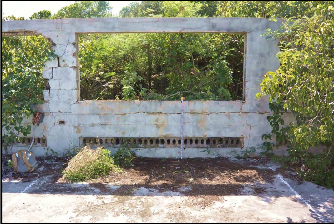
Figure 12: Photograph of south wall details, note the large window openings and ventilation features near the base of the wall
