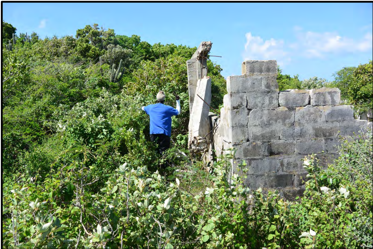
Figure 3: Photograph of hand clearing of vegetation to expose the exterior of Building A south east corner wall
