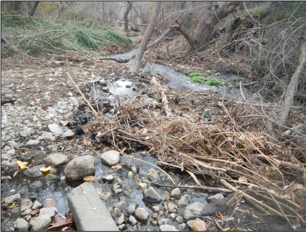
Figure 7. Dam blocking Haines Canyon Creek near the West Pond on January 18, 2016.
