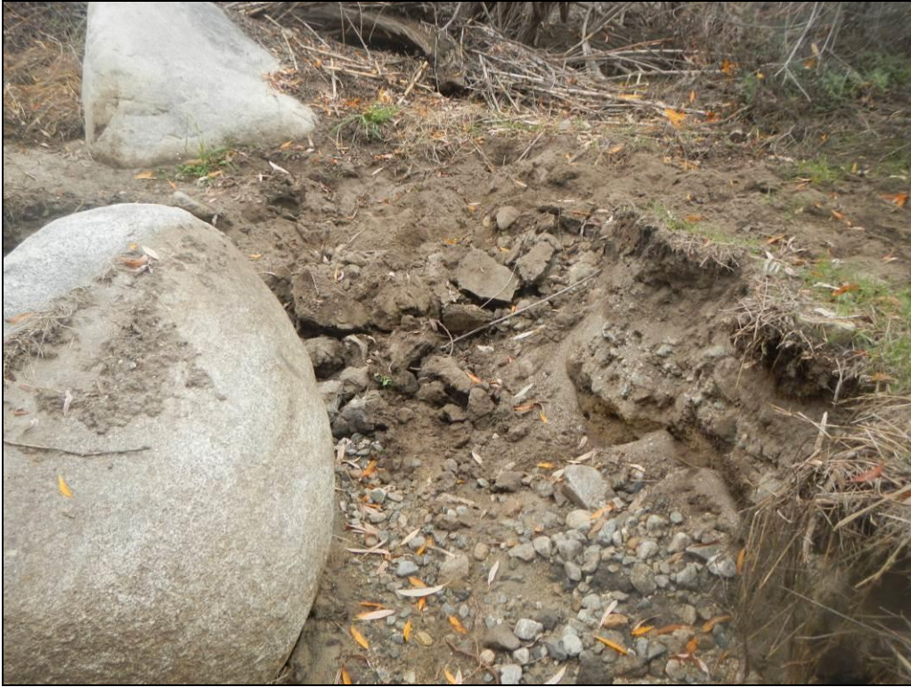
Figure 13. Eroded trail between the Cottonwood Gate and Haines Canyon Wash. Photo was taken facing east at the north-south oriented trail on January 18, 2016.
