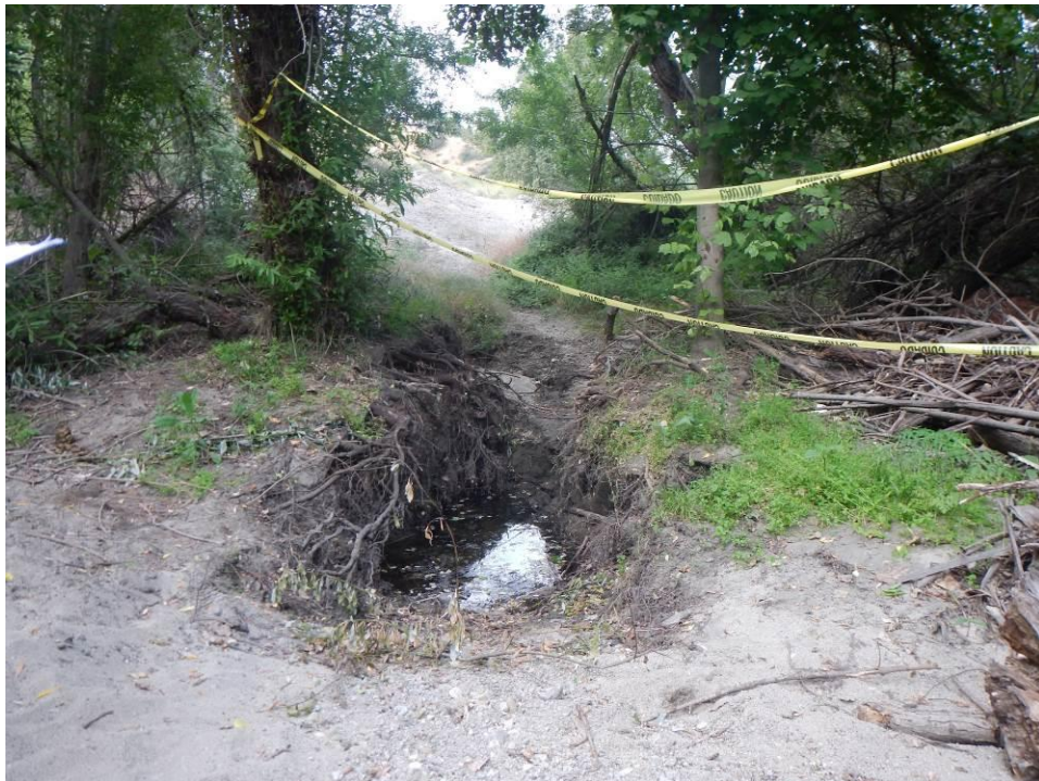
Figure 7. Heavy erosion causing stagnant water.
