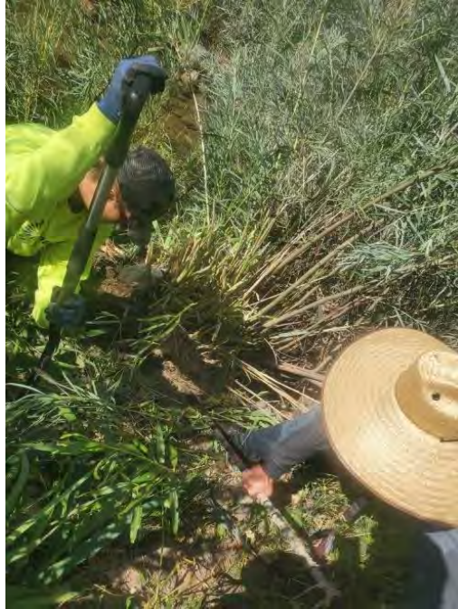
Photo 7. Removal of giant reed found in Big Tujunga Creek, on July 10. This large perennial species has an extensive rhizome which must be fully removed to prevent re-sprouting.
