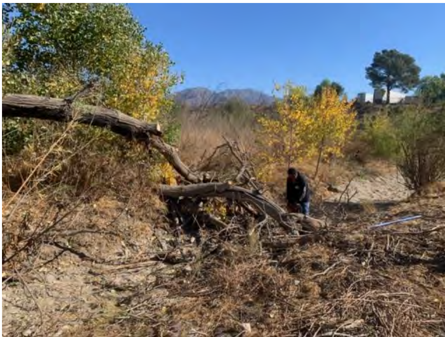
Photo 4. The crew used a chainsaw to cut the tree snag into smaller segments, on December 14.
