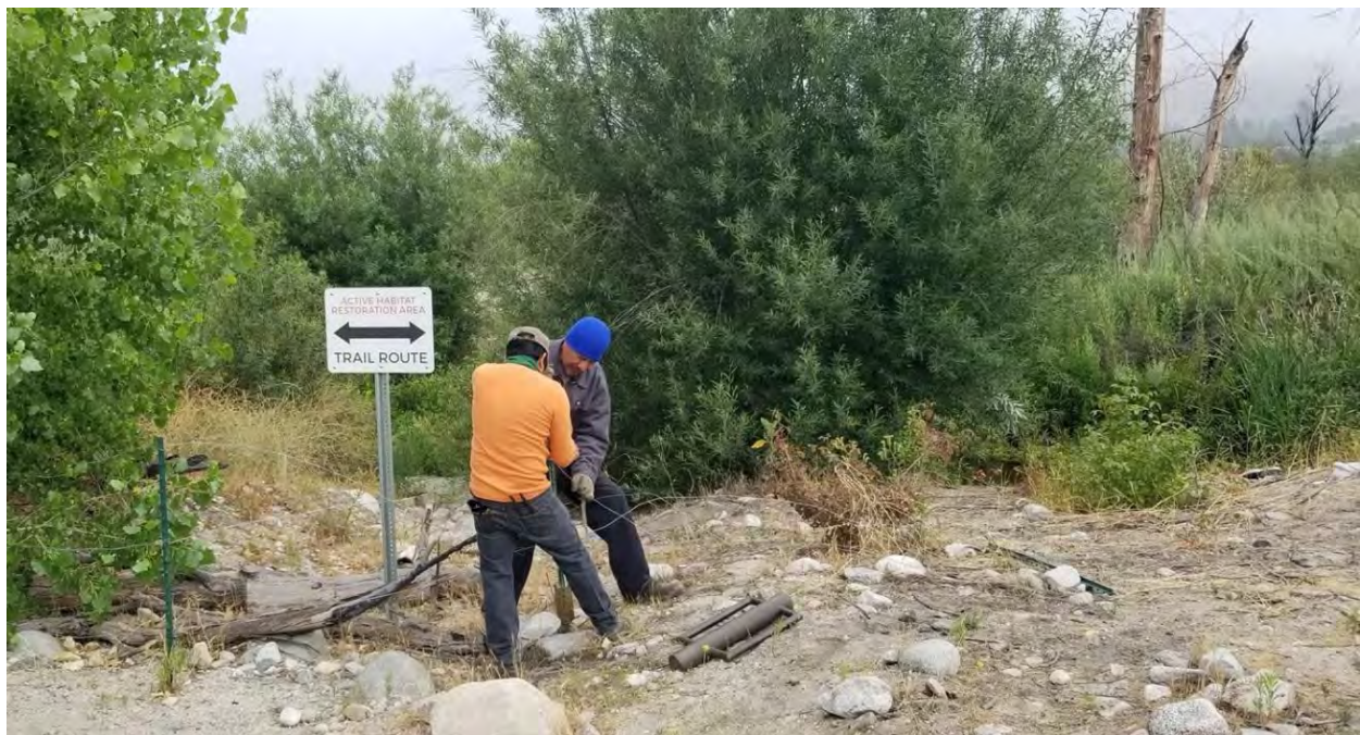
Photo 10. Crew members repairing the vandalized creek crossing closure, resetting T-posts, and replacing the wire fencing, on June 26.
