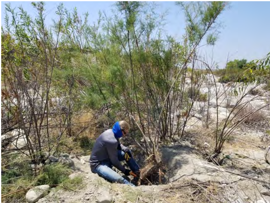
Photo 8. Removal of Mediterranean tamarisk found in Big Tujunga Creek, west of the 210 freeway embankment and property boundary, on August 11.
