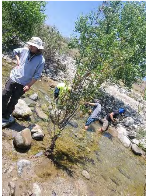
Photo 9. Crew members disassembling a dam constructed across Big Tujunga Creek during exotic species removal efforts, on May 27.
