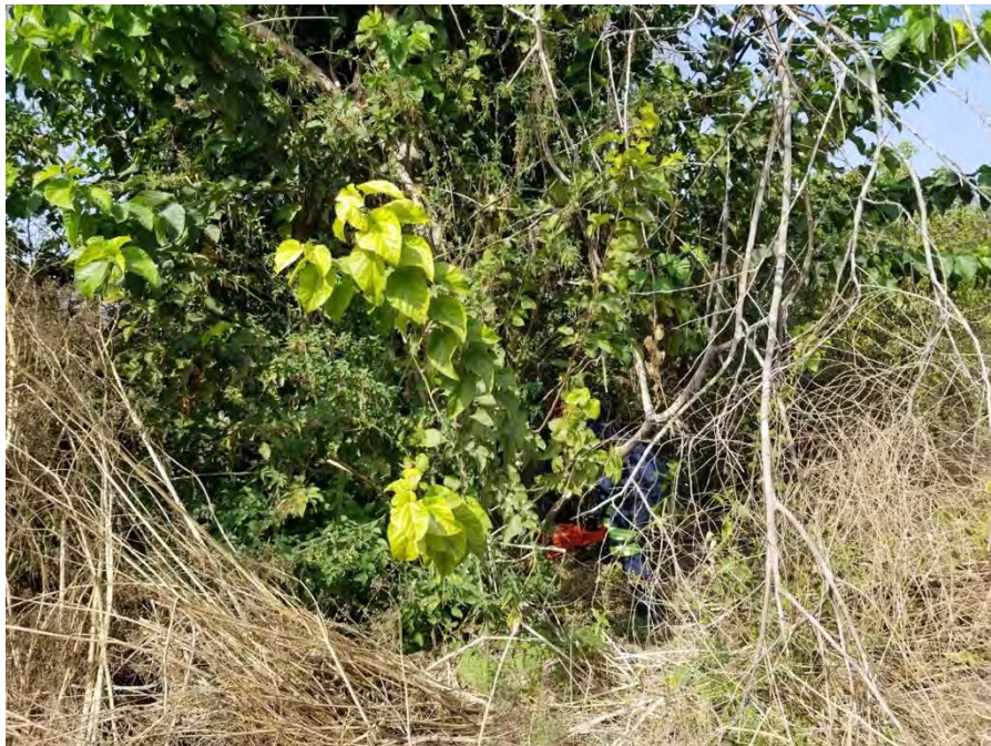
Photo 12. The crew used chainsaws to cut a white mulberry that grew intertwined with a native tree, on October 9.
