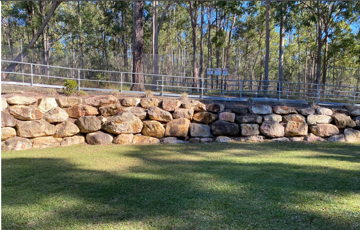
Figure 5-11 Interface with Western Boundary of the College (Army Barracks) Source: Urbicus site photos
