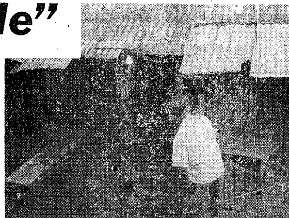
DARK AND IN FINAL stages of deterioration, these houses are homes of Waipahu workers. The workers keep the interior as neat and livable as possible but plumbing is bad and the kitchen area is damp from open sewers. Rats infest the area.
