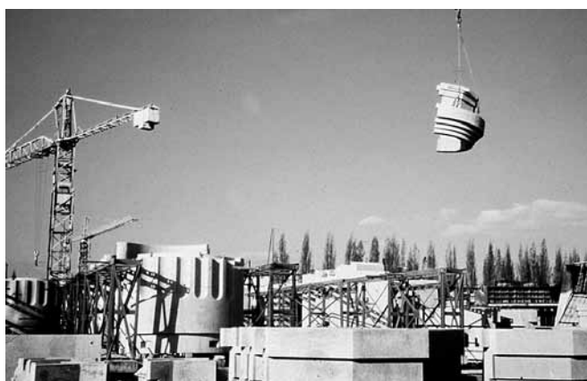
Figure 2. Construction site of Abraxas 1982-1983. (Courtesy of Ricardo Bofill – Taller de l'arquitectura, Barcelona)
