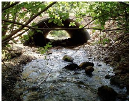
Figure 36. Example of a culvert that is a barrier to aquatic organism passage (© Wikipedia), and a culvert that can pass aquatic organisms (© USFS).
