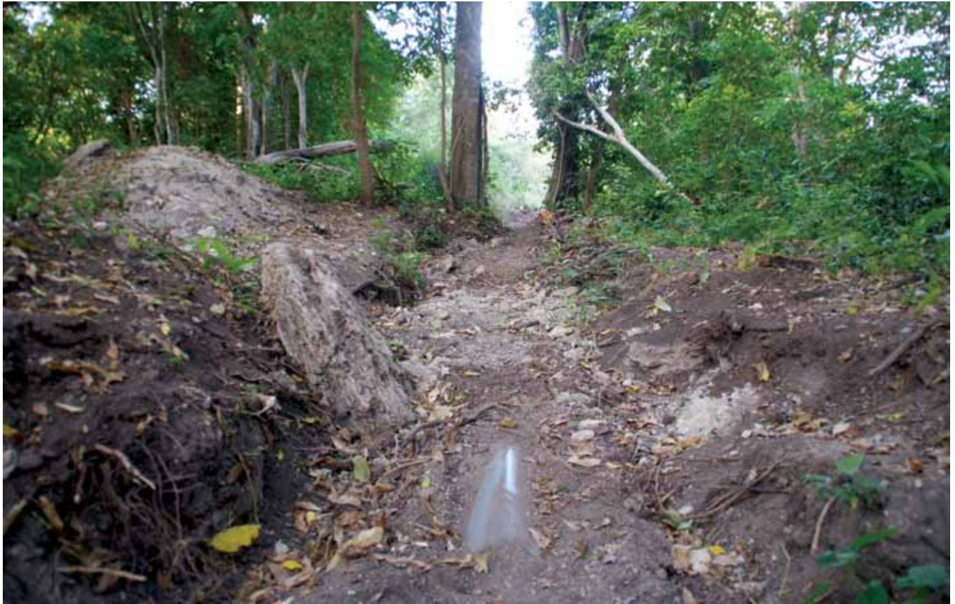
The laying of the new pipeline involved breaking the rock layer that is possibly a key feature of the functioning of the system.
