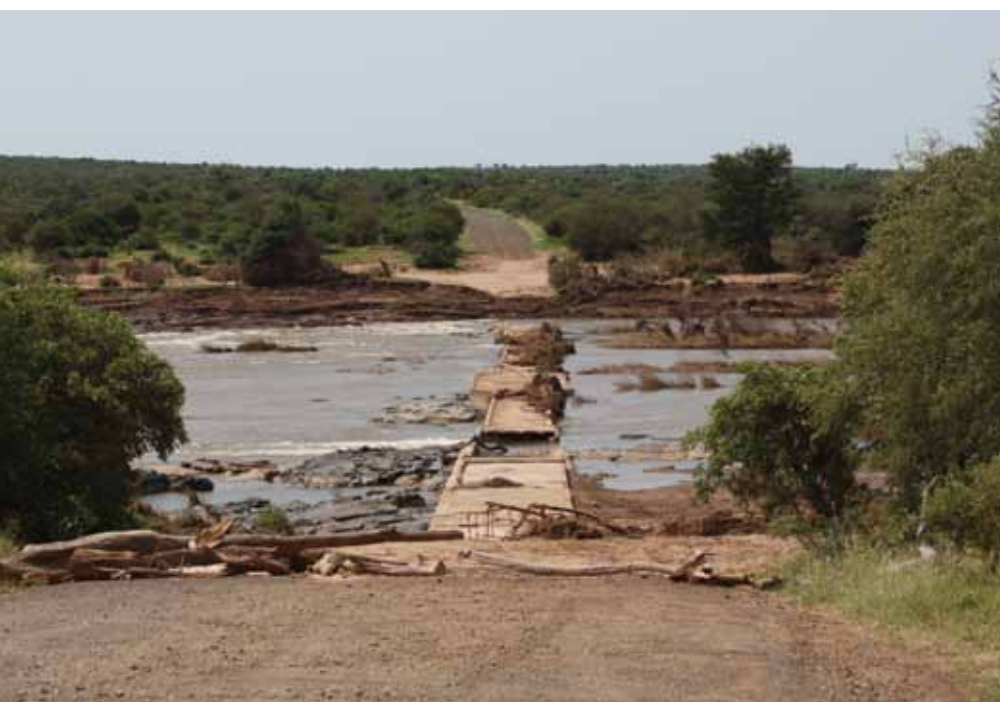
One of the causeways damaged by flooding.
