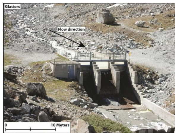
Figure 1: a classic Alpine water intake (Lower Berthol, Valais, Switzerland)
