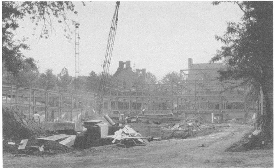
I&LR School Buildings Take Shape —On the former site of James Law Hall at East Avenue & Tower Road, steel is rising for the $2,755,000 plant of the School of Industrial & Labor Relations. The former Veranus A. Moore Laboratory, at right, and the former Veterinary College buildings in the background, along Garden Avenue, are being remodelled for the I&LR School's new Campus, scheduled for occupancy in September, 1961. Photo Science
